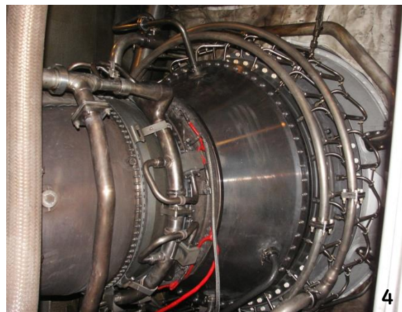
LM1600 Power Turbine
